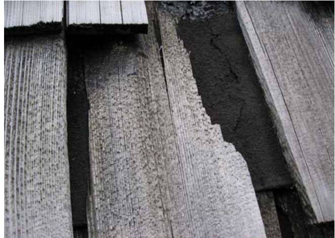
Shingles on the Cabin Roof. They are 25 years old. We had them evaluated and the experts said they were near to the end of their life.
